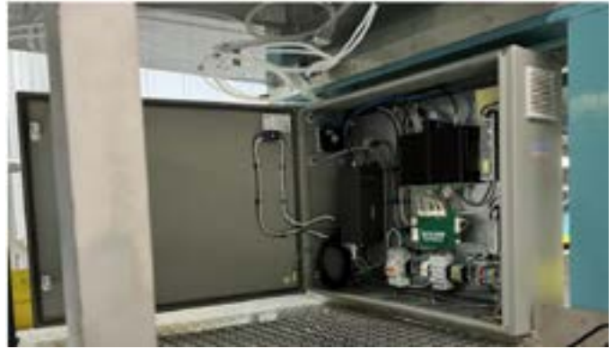
The control panel for the wrinkle detection system. Source: Vision Optronix/Teledyne Dalsa
